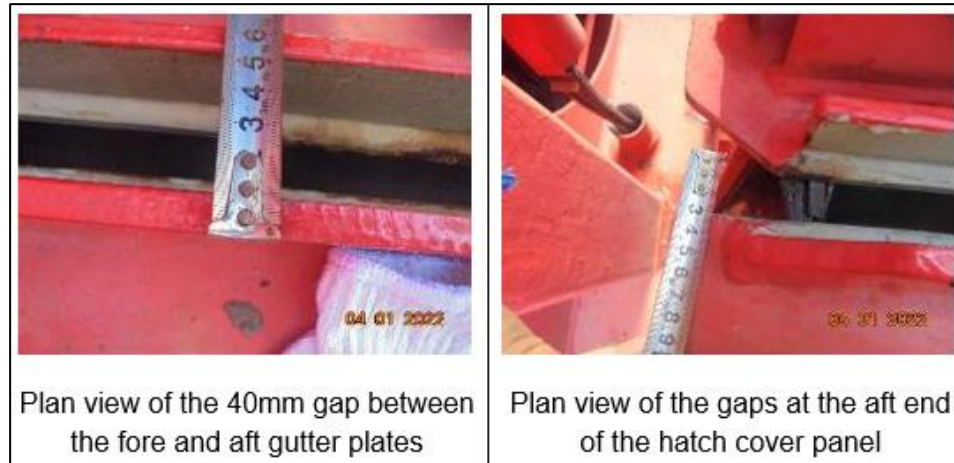
Figure 23 - Gaps between the hatch cover panels - Source: The Company
