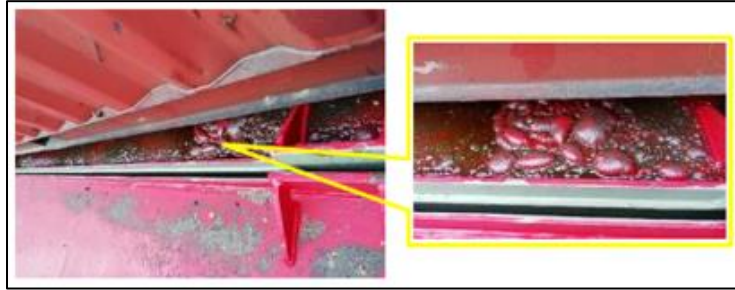
Figure 2 - Bubbling of hatch cover paint underneath container FSCU7712264 - Source: The Company (annotation in yellow by TSIB)
