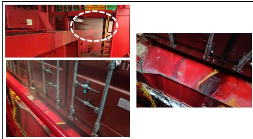
Figure 4 - Orange/ brown 45 smoke and acid leak as reported by the Master - Source: The Company ( annotation by TSIB )
