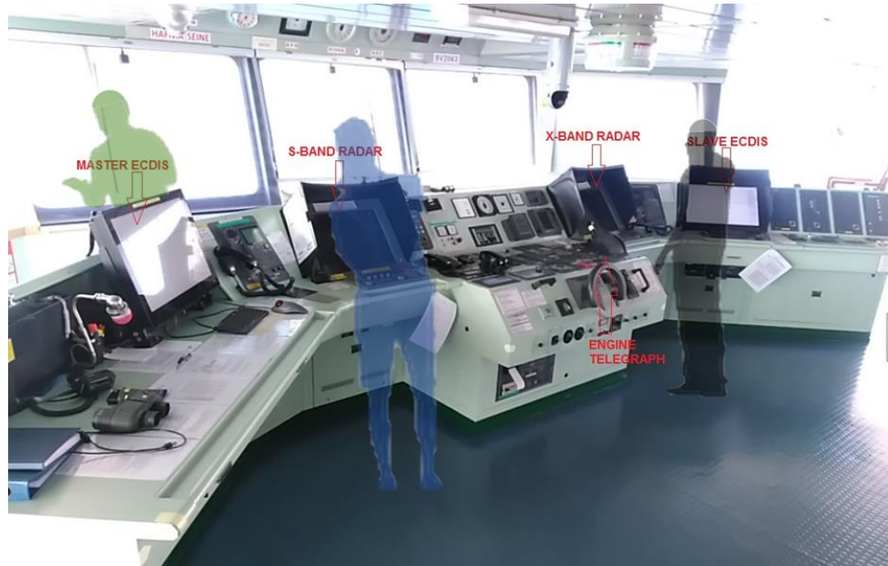
Figure 7 – SE's bridge view, looking forward (as viewed from the port side), with the positions of Master (black), ASD (green, performing the role of a lookout) and 2O (blue) (Source: the Company – annotations by TSIB)
