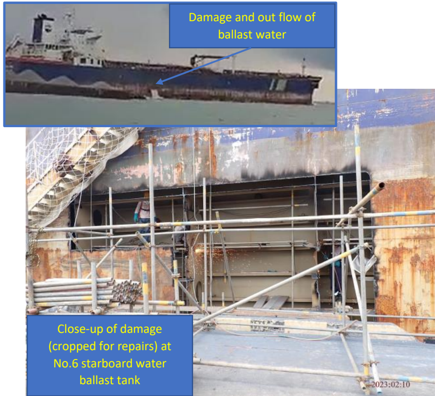
Figure 18 – Hull damage on SE ( Source: the Company and SOL1 (inset) – annotation by TSIB )
